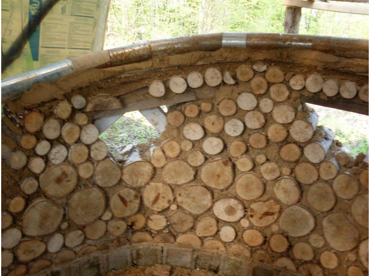
A cordwood wall. London Permaculture photo, published under the Creative Commons licence.
