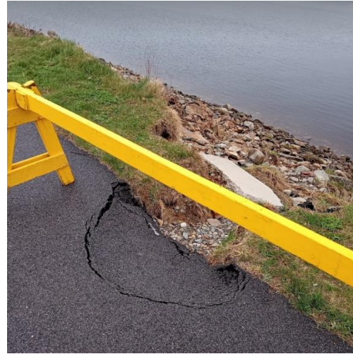
Picture 2 – Damage to Coastal Link Trail after storm surge (2024)
